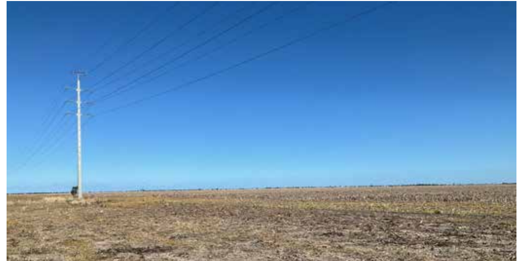
Existing overhead electricity network in the southern areas of the precinct Courtesy of Rhelm
