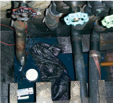
Dirty oil contaminated bilge
