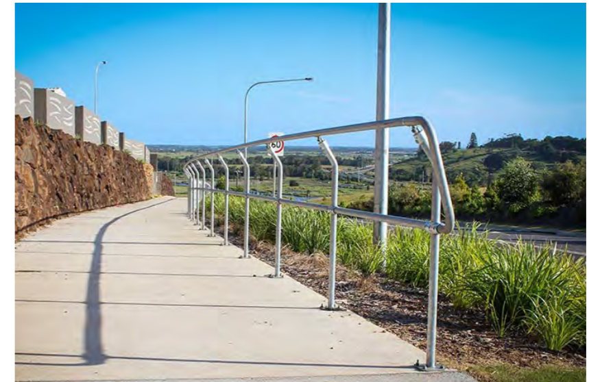
Figure 55. Pedestrian and cyclist safety fence with deflection rail
