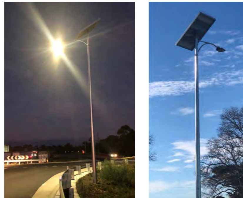
Figure 50. Shared path lighting pole, outreach arm and solar panel
