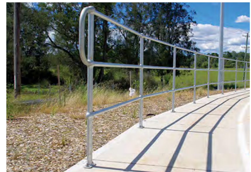
Figure 56. Pedestrian safety fence - Monowills
