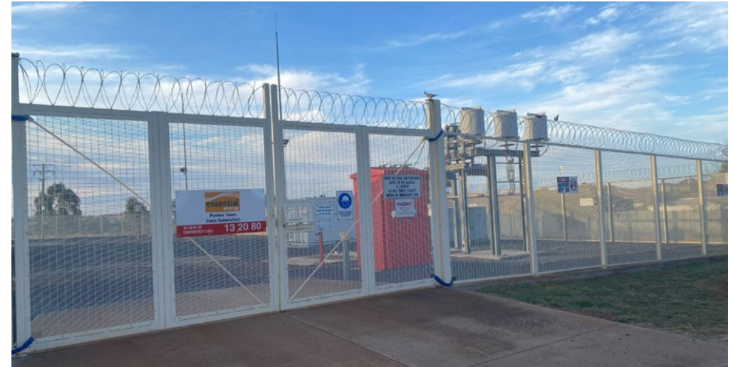
Essential Energy substation
