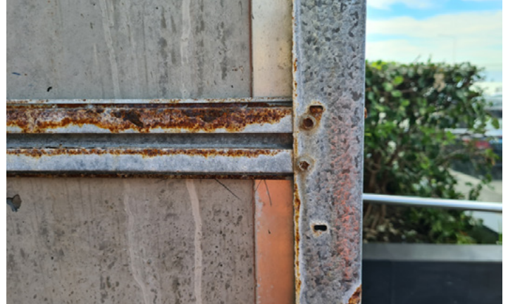
Figure 5.5: Care must be taken with products formed from galvanized sheet to prevent corrosion
