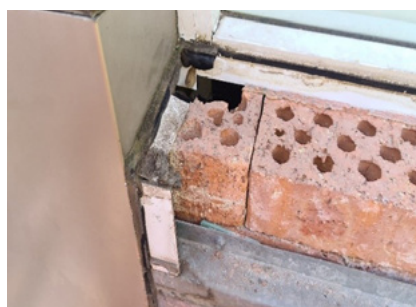
Figure 15.6: Inadequate wall structure
