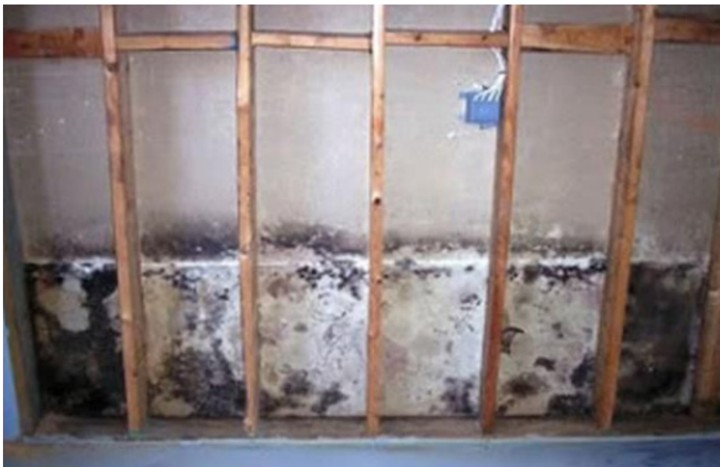
Figure 11.1: Black mould growth in a wall cavity due to poor ventilation and condensation on inside face of cladding
