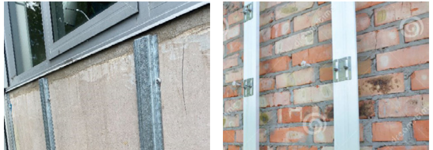
Figure 15.9: Inadequate or lack of insulation
