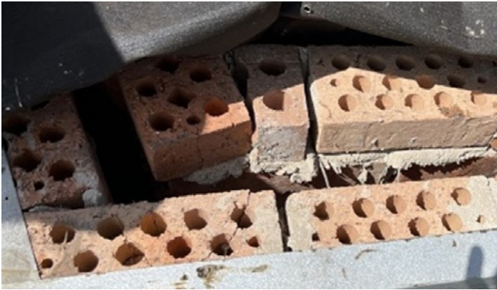
Figure 18.5: Defective masonry construction
