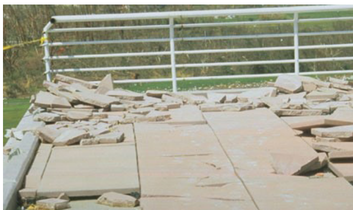
Figure 14.8: Paver uplift damage during Hurricane Andrew in Miami. (after Tom Smith)
