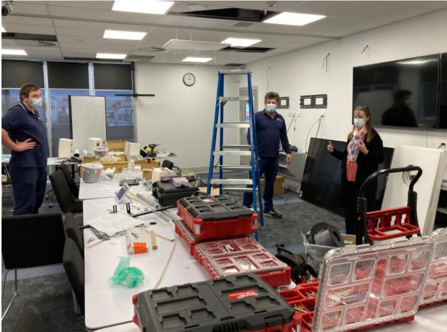
Sharyn Cowie (Manager, Telehealth, Health ICT) discussing with Tom Mugridge (left) and Andrew Lazar of Syndeticom (Sydney-based tech company) about the new equipment being installed in the CHC auditorium.
