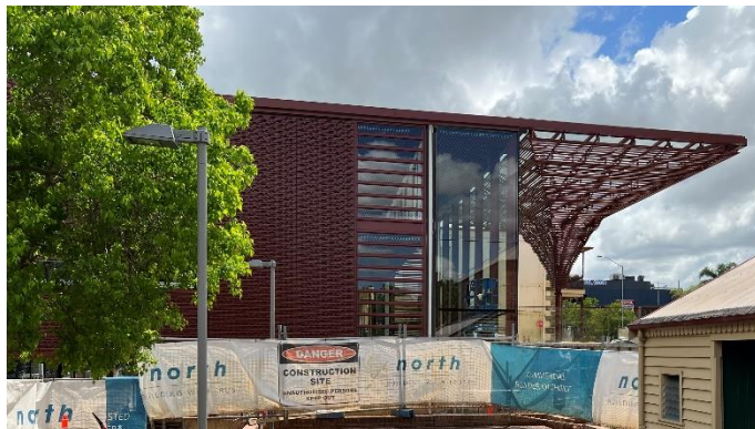
Figure 18: Construction of the Donald Horne Building, home of the Upper Hunter Innovation Precinct. Photo credit: Muswellbrook Shire Council.
