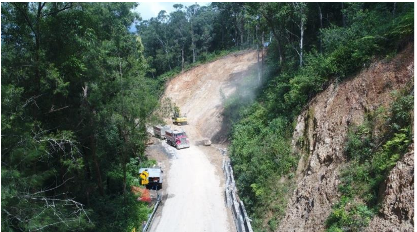
Figure 20: Thora landslide repair works underway on Waterfall Way. Photo credit: Bellingen Shire Council.
